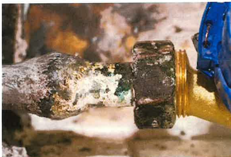
An old lead service line is attached to this water meter.
