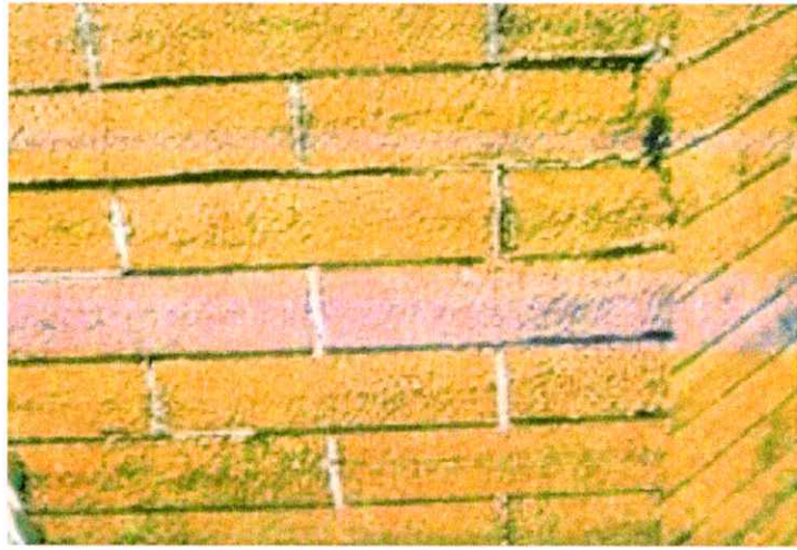
Sandblasting brick or stone as a method of cleaning permanently erodes the surface of the material and accelerates deterioration.
